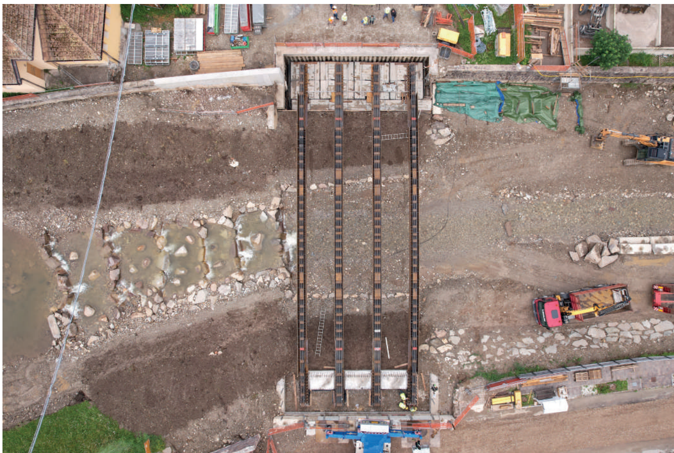
△ The new bridge with a single span of 25.6 metres and a width of 11 metres.
