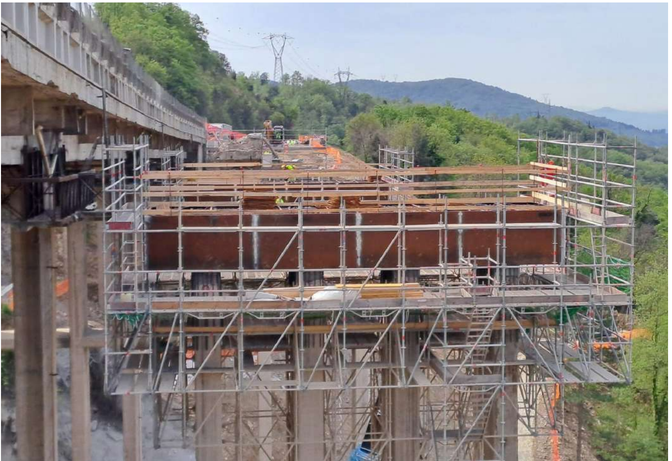
△ Bridge bearings on the Torraccia Viaduct – A1 MI-NA motorway.
