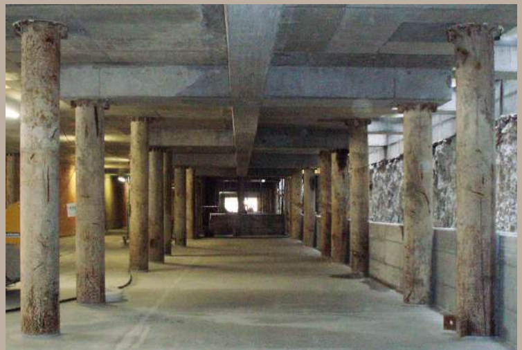
△ NPS® columns and NPS® beams used to build the site from ground level down.
